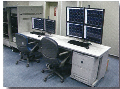
振動監視装置 (Vibration Monitoring System)
