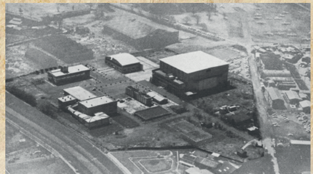
LEFT: Transonic wind tunnel during foundation works, photographed in 1958. The general shape of the closed circuit wind tunnel is visible.
