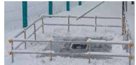
The snow and ice monitoring sensor installed at Kitami Institute of Technology (Top: Construction in progress; Bottom: Installation site)
