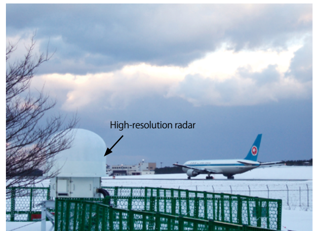
Fig.2 ● High-resolution radar installed at Shonai Airport
