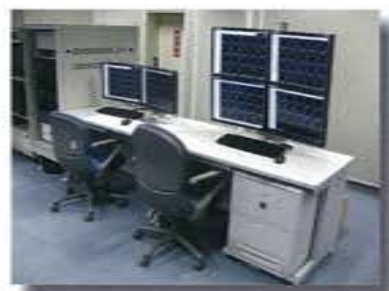
振動監視装置 (Vibration Monitoring System)
